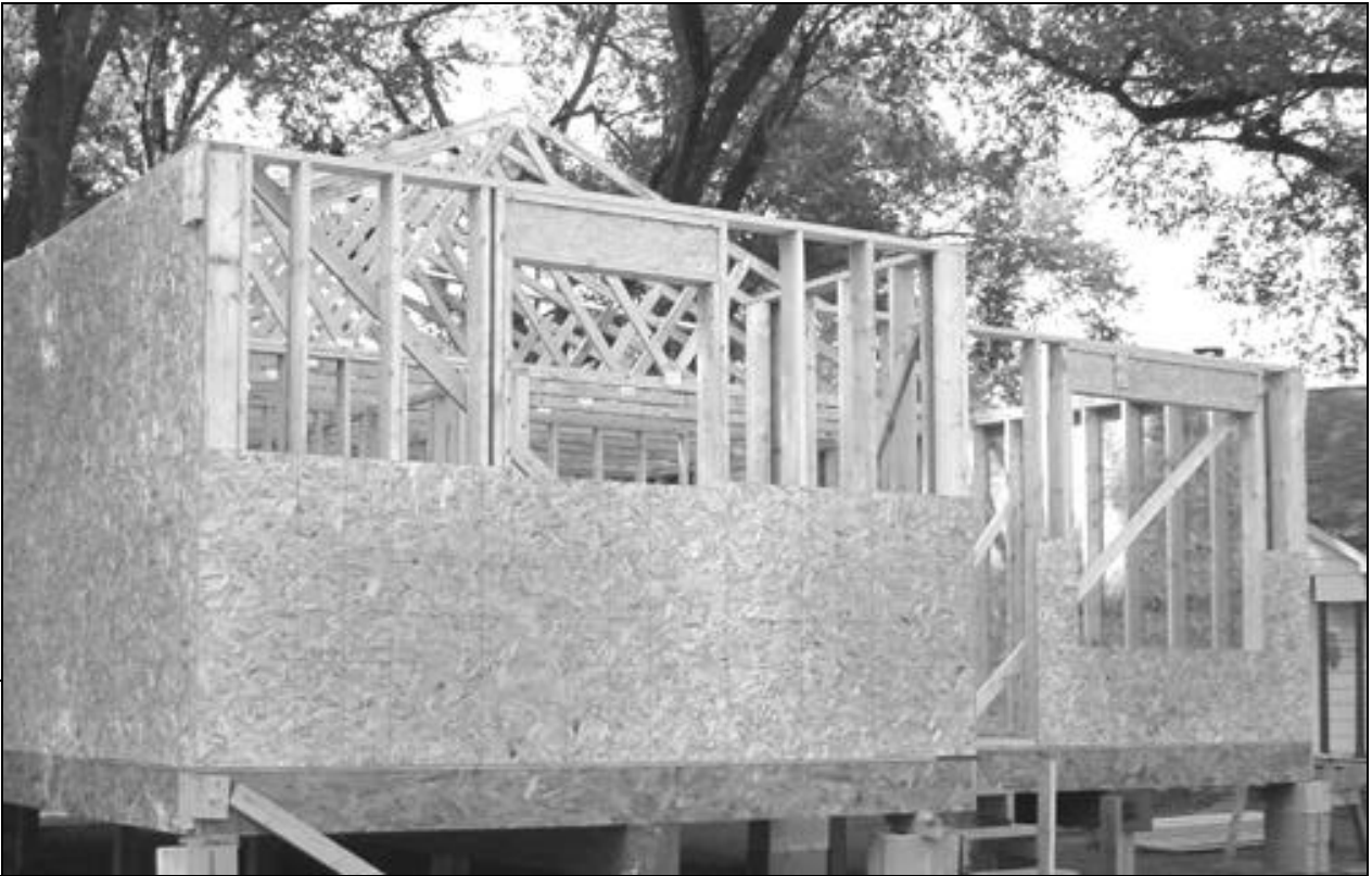
Photo courtesy Habitat for Humanity Work on the Rose-Hulman Habitat for Humanity house continues with the addition of particle board that will allow the house to shed water.
