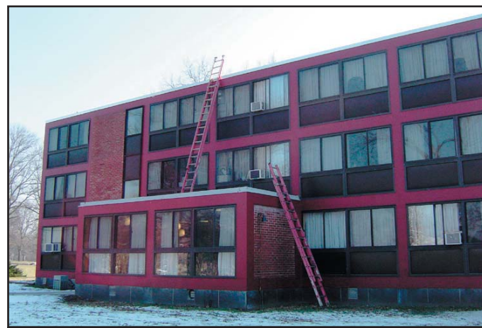
Matt Durham / Photographer Speed has required several construction projects just this year, including roof work, window resealings, and painting.
