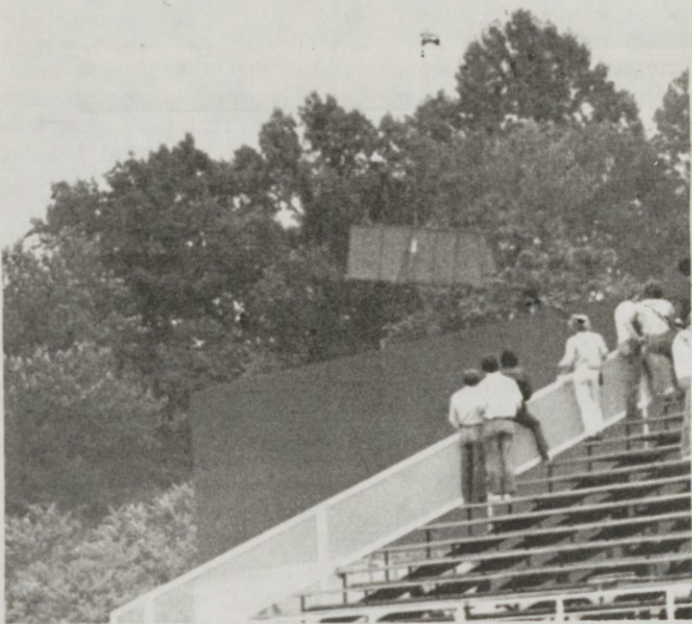
A crew from St. Louis Helicopter Airways, Inc., lowers a one-ton air control unit to the roof of the new recreation building. Placing the six units was done in 25 minutes — a "piece of cake" for the sure young workmen.
