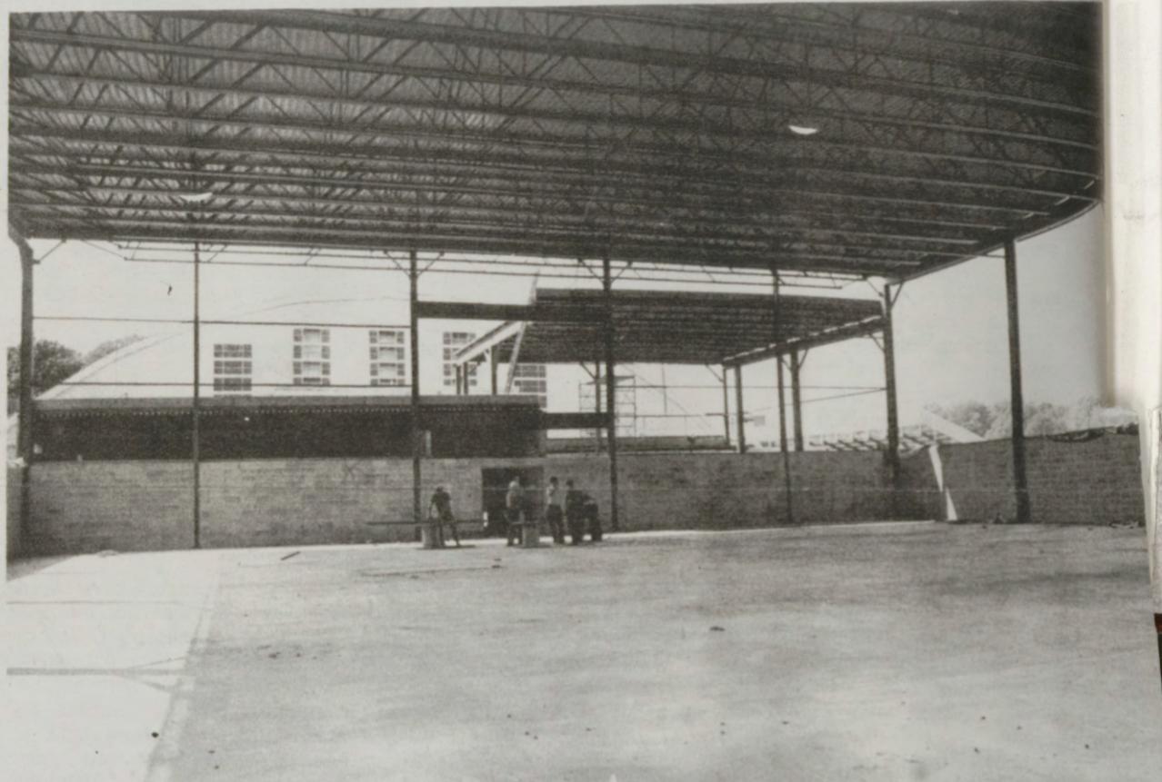
The gymnasium portion of the Recreation Center as viewed from the east court. A multipurpose room and handball/squash court area are sited between the gymnasium and east end of Shook Fieldhouse.
