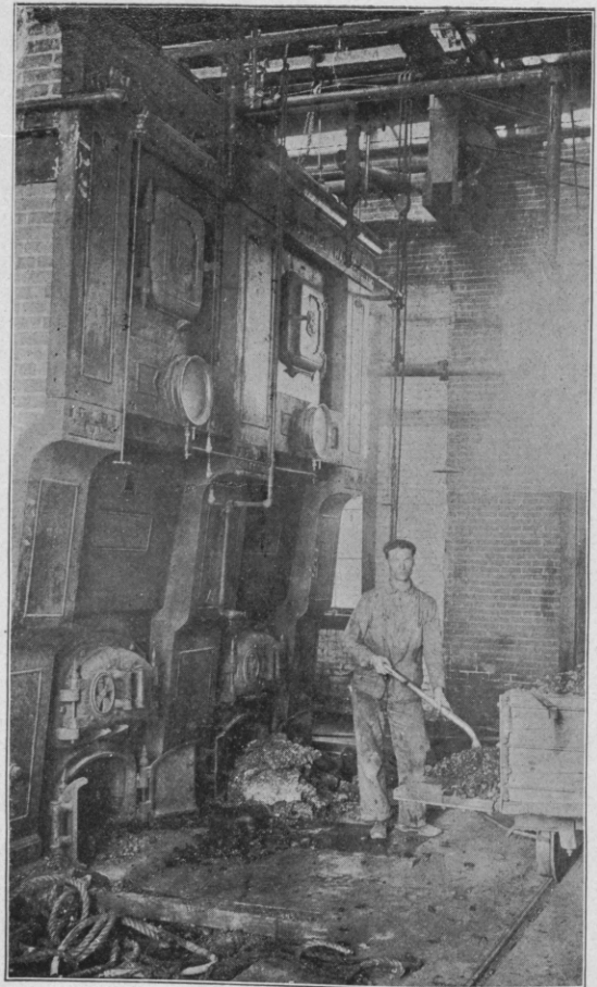
THE NEW BOILERS, JUST AFTER COMPLETION.
