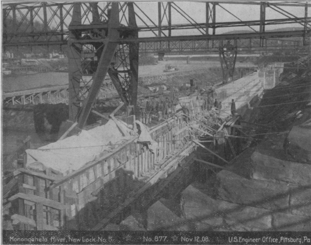
The land wall of the lock partially completed and the forms to shape the concrete, also a close view of the cranes.
