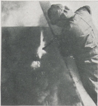
LIKE CUTTING CHEESE —the oxy-acetylene cutting blowpipe demolishes a 52-ton cast iron rock crusher bowl.
