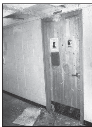
Nathan Ingersoll/ Guest Photographer A jet of water from the broken sprinkler hits the top of the door of room 209.
