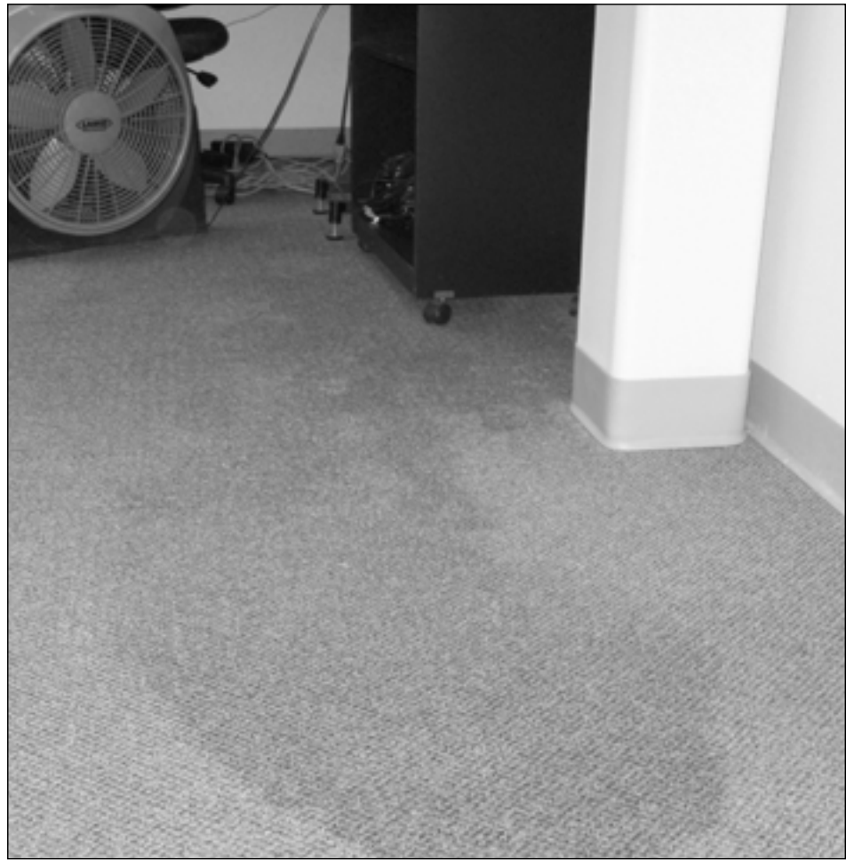
Even with extensive renovations this year, the lower level of the Logan Library still experienced some groundwater leaking during the heavy April showers.
