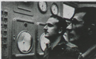
Beverly, Ohio — TEST ENGINEER Norman Blair taking readings in the control room of a 430,000-kw generating plant.
