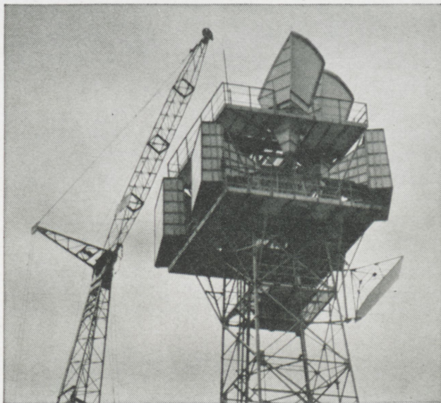
Microwave relay towers assure reliable land transmission of telephone, radio, television and data traffic—with complete flexibility.
